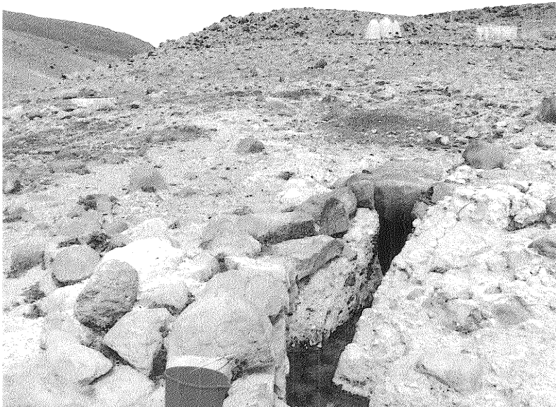
The outlet of the qanat in Shallalah Saghirah in northern Syria, which supports the village with sustainable water flow for domestic and agricultural use round the year.
