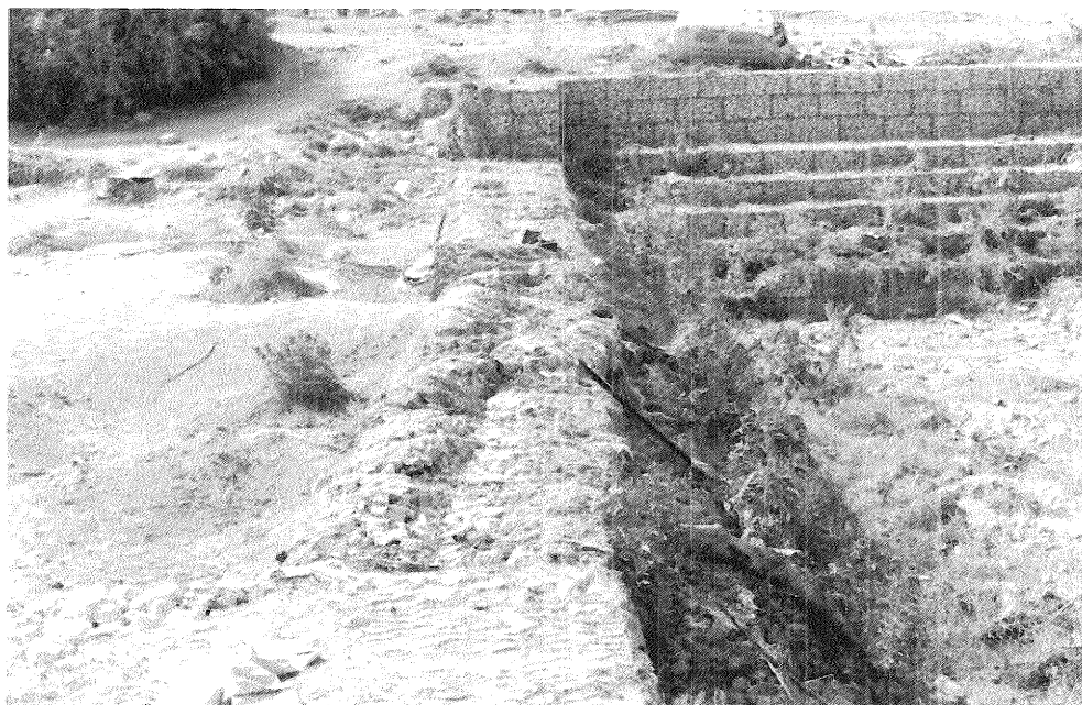
A gabion dyke erected on Wadi Suk Alkhamis, for water spreading and flood protection.
