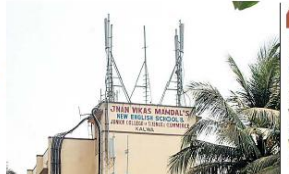
TELECOM PLANS: Government is trying to work out solutions to solve the problem of health hazards due to mobile towers
