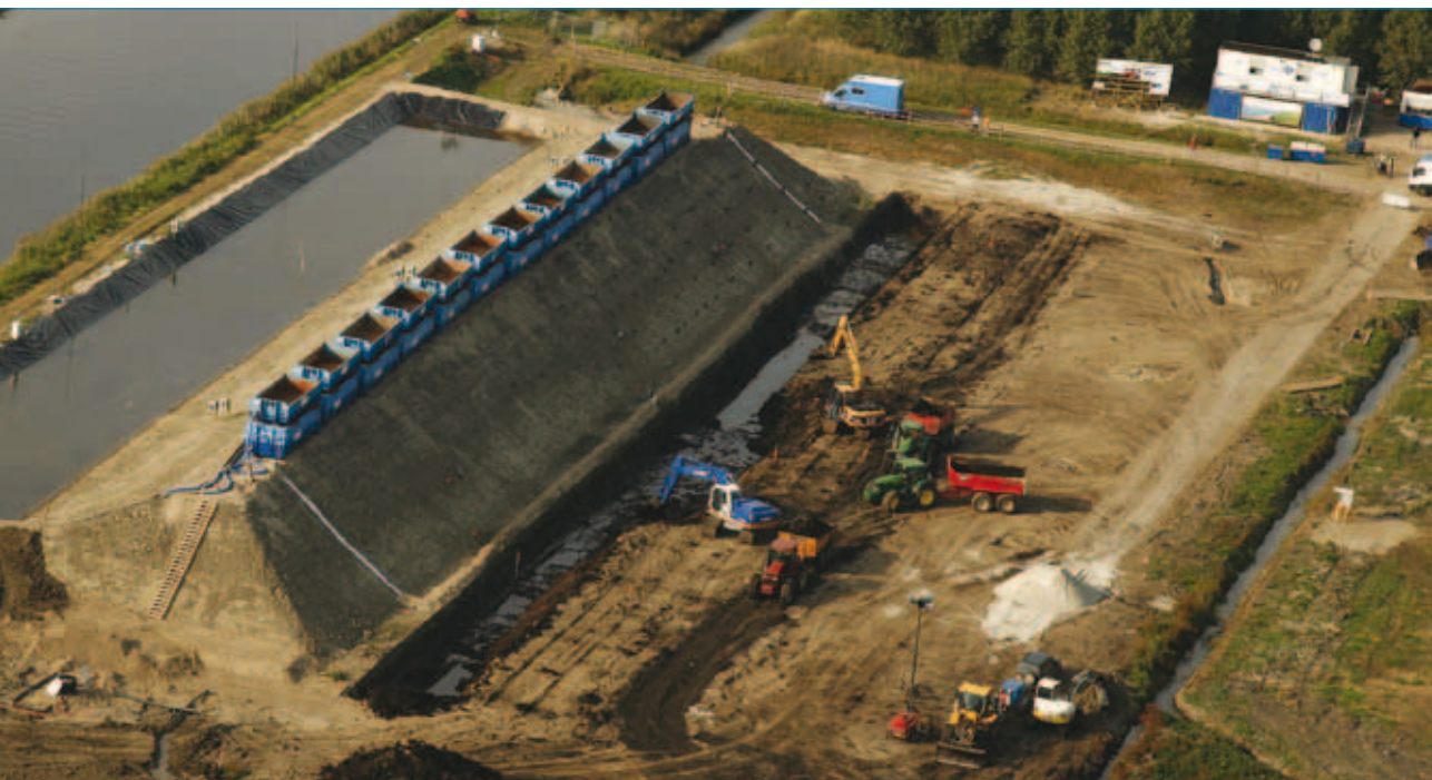
Construction of the Smart Dike that was brought to failure in the Macrostability Experiment conducted in September 2008 (see also photo on page 28)
