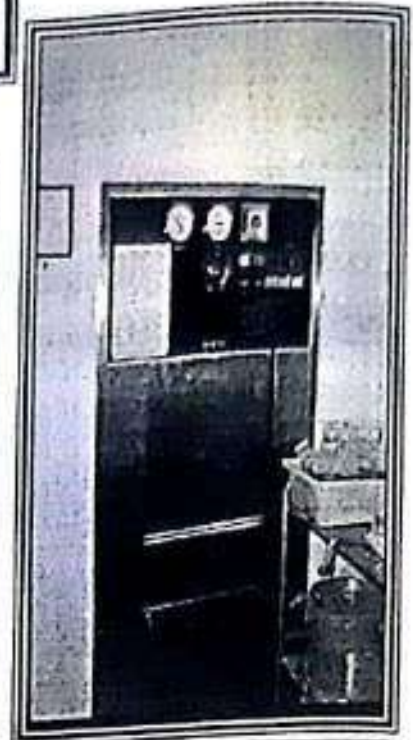
large, front-loading (boiler outside wall)
