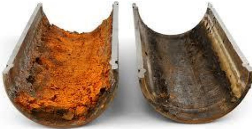
Figure (1-1) corrosion of piping
