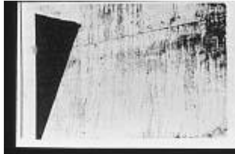
Honey combing- Sand streak-loss of cement grout from the form
