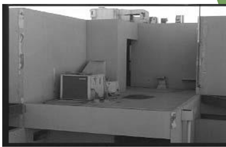
A/C unit on the roof- Without proper design for drainage
