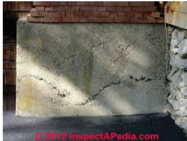
Cold joints Due to pouring concrete in different times
