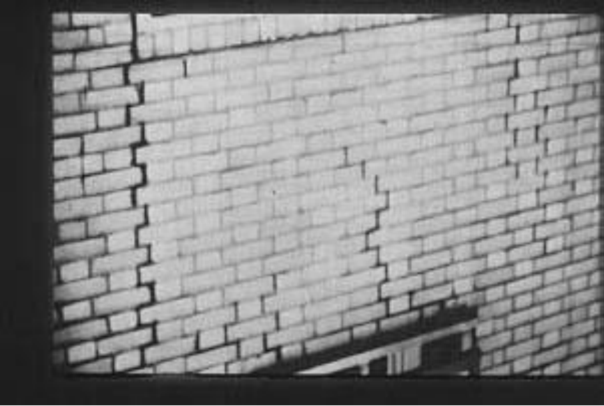
Wall cracks- Poor detailing-strong bond - vertical crack
