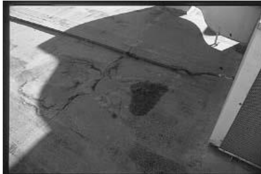
unit on the roof- Without proper design for drainage
