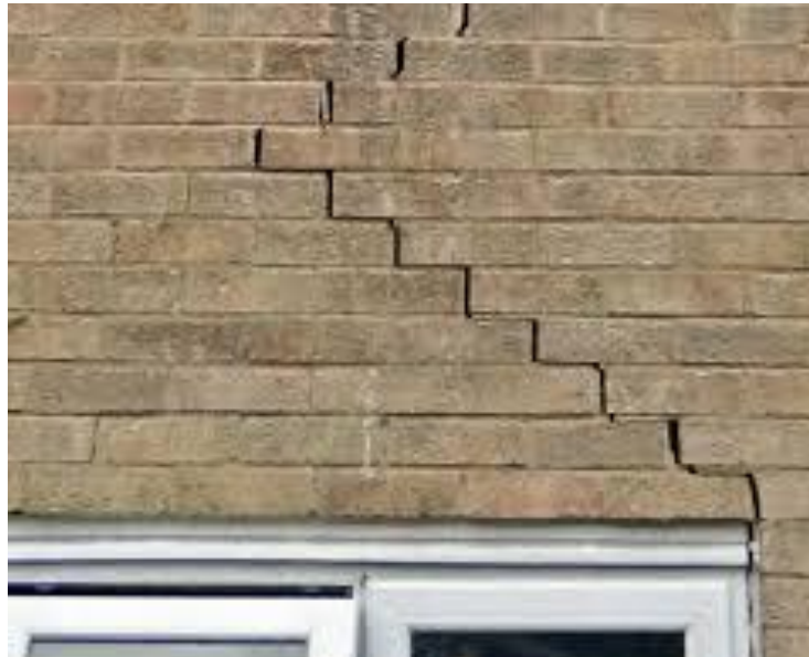
External wall- Diagonal Cracks
