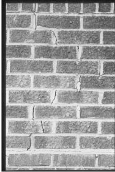
Wall cracks- Poor detailing-Diagonal crack- Expansion and shrinkage
