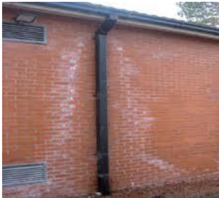
External Finishing presence of moisture in between-
