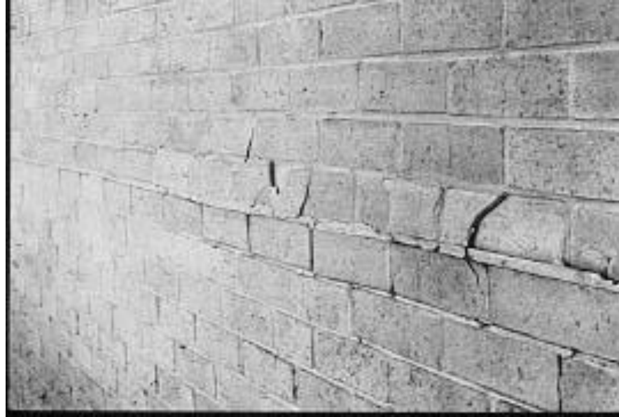
External wall -Poor detailing-Spilling of brickwork cladding-compression of the
