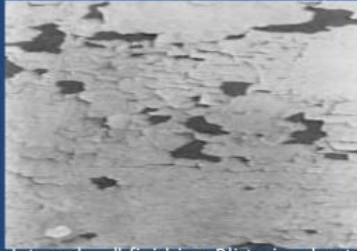
Internal wall finishing: Blistering due to dampness-chemical-water vapour
