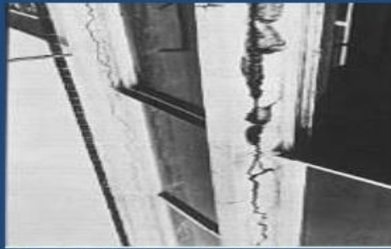
Corrosion Workmanship-inadequate concrete cover
