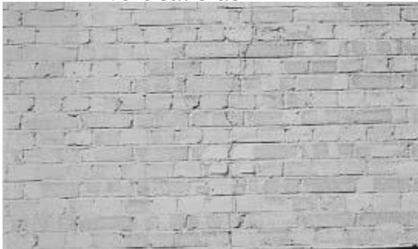
Wall cracks- Vertical crack-cavity clay brick work- restrained by columns
