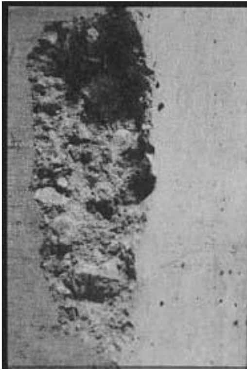
Sticking to forms Damage caused during stripping of formwork from concrete
