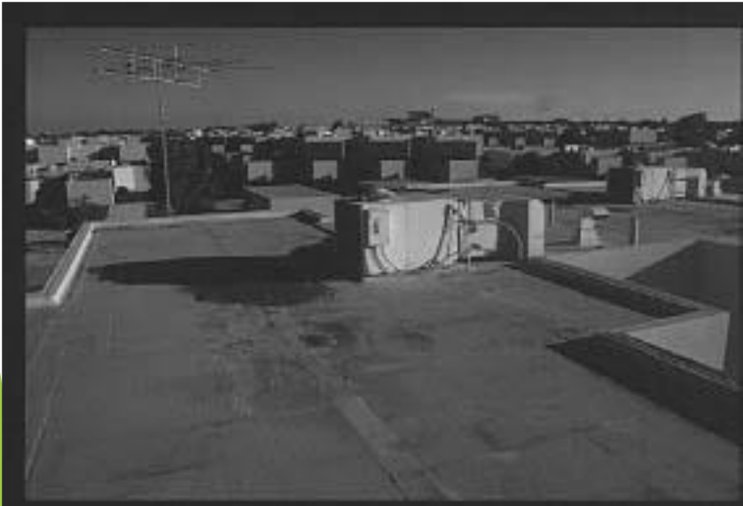
A/C unit on the roof- Without proper design for drainage-
