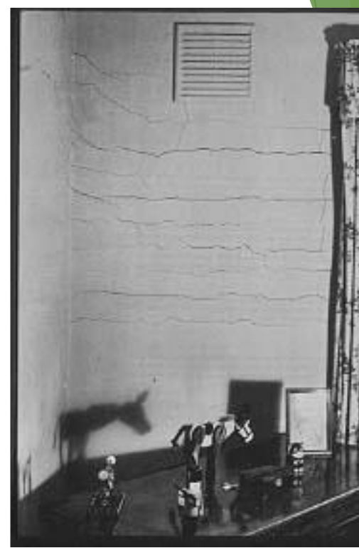
Internal Finishing :plaster Cracks due to shrinkage-base wall movement use different materials
